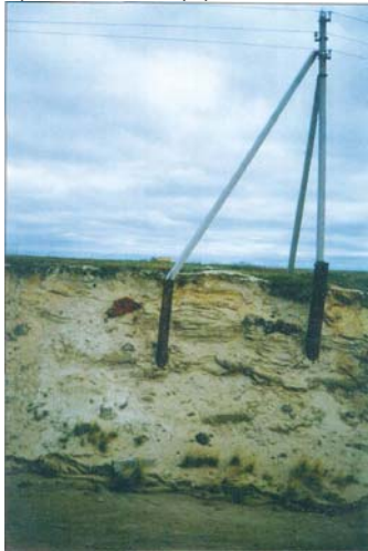
Photo 7. Thermoerosion also intensifies in cases of human-related breaching of vegetation cover. The construction of a pipeline and parallel power line triggered thermoerosion processes along the pipeline, which threatened the balance of power transmission towers (Photo credit: A.N. Kozlov, Department of Geocryology, Moscow State University, Russia)
