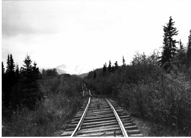
Photo 4. Thermokarst poses a formidable threat to railroad maintenance. The photo illustrates the numerous deformations of the Northwestern Railway near Strelna, 75 miles northeast of Valdez, Alaska (United States). The thermal equilibrium of the fine-grained sediments underlying the roadbed was disrupted during construction, and the permafrost started to thaw differentially. Maintenance and use of the railroad were discontinued in 1938. Subsidence, as well as lateral displacement, has continued (Photo credit: U.S. Geological Survey, September 1960)
