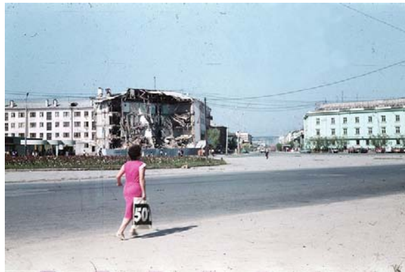
Photo 3. The photo shows a wall collapse in a dwelling in Yakutsk, Russia, caused by thermokarst. Nobody was injured. To prevent such collapses, houses must be built on piles. Hereby, the air space under the house should prevent the heat impact on the frozen ground. This house was erected ‘low-sitting’, and for the long time it was occupied, the air space became stuffed with finely dispersed material. This led to gradual melting of frozen grounds lying below (Photo credit: Y.A. Murzin, Institute of Permafrost Studies, Russian Academy of Sciences, July 1993)
